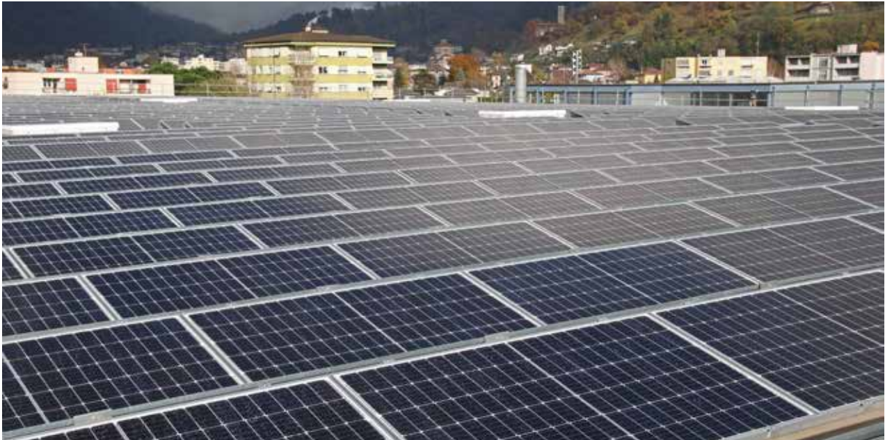
Photovoltaic plant, Raiffeisen BiascaArena, Biasca, Switzerland.
