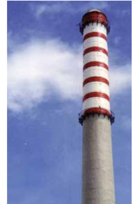
Aircraft warning colors using SikaCor® EG 5 as the top coating in zone 1 of a concrete chimney refurbishment.
