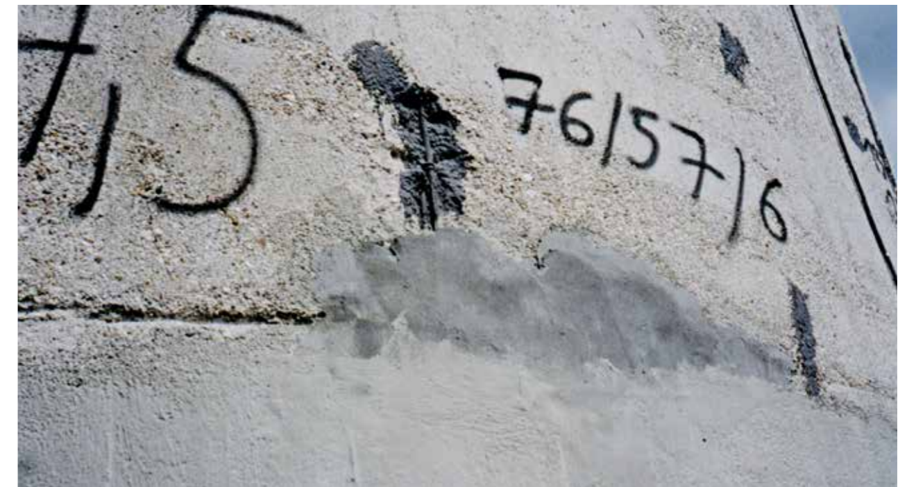
Steel reinforcement prepared and protected with Sika MonoTop®-910 ready for repair mortar application.
