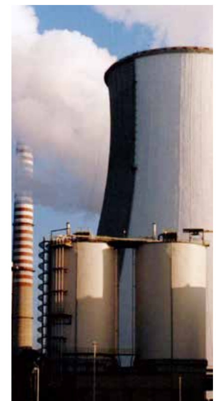
Sika protective coatings being applied to the external surfaces (all zones) of a cooling tower.
