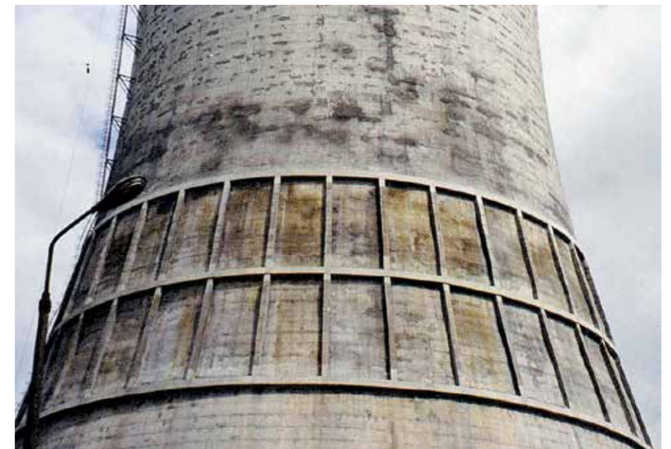
Carbonated concrete with spalling over corroded reinforcement accelerated by the steel being attacked by the acidic exhaust gases.
