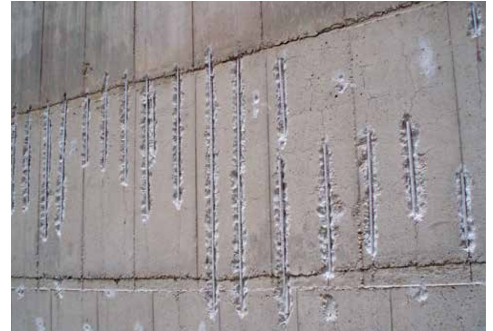
General corrosion induced by carbonation aggravated with low concrete cover issue.
