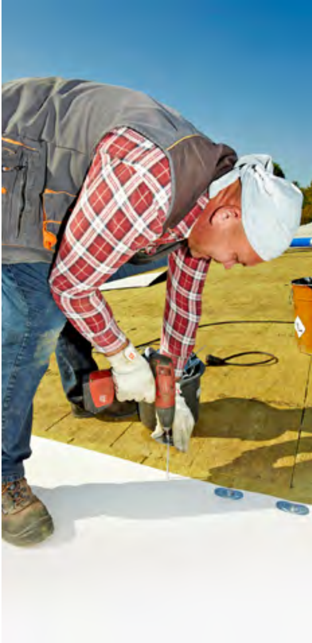
1989 | Sarnafast® spot fastening in overlapping mechanically fastened roof systems was introduced to resist wind uplift and for increased speed of installation.
